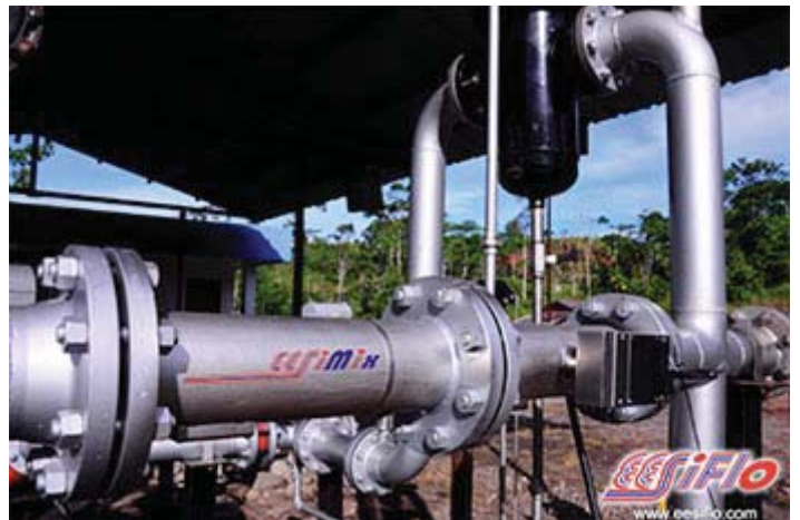
Crude Oil Export Metering Stations
