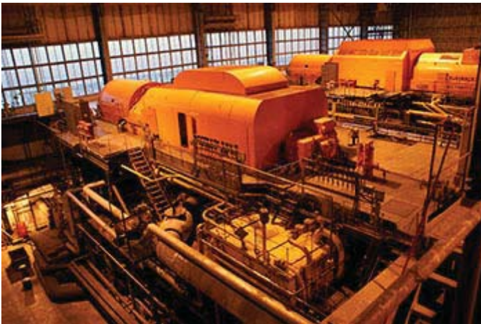
Power Plant – Power Production
